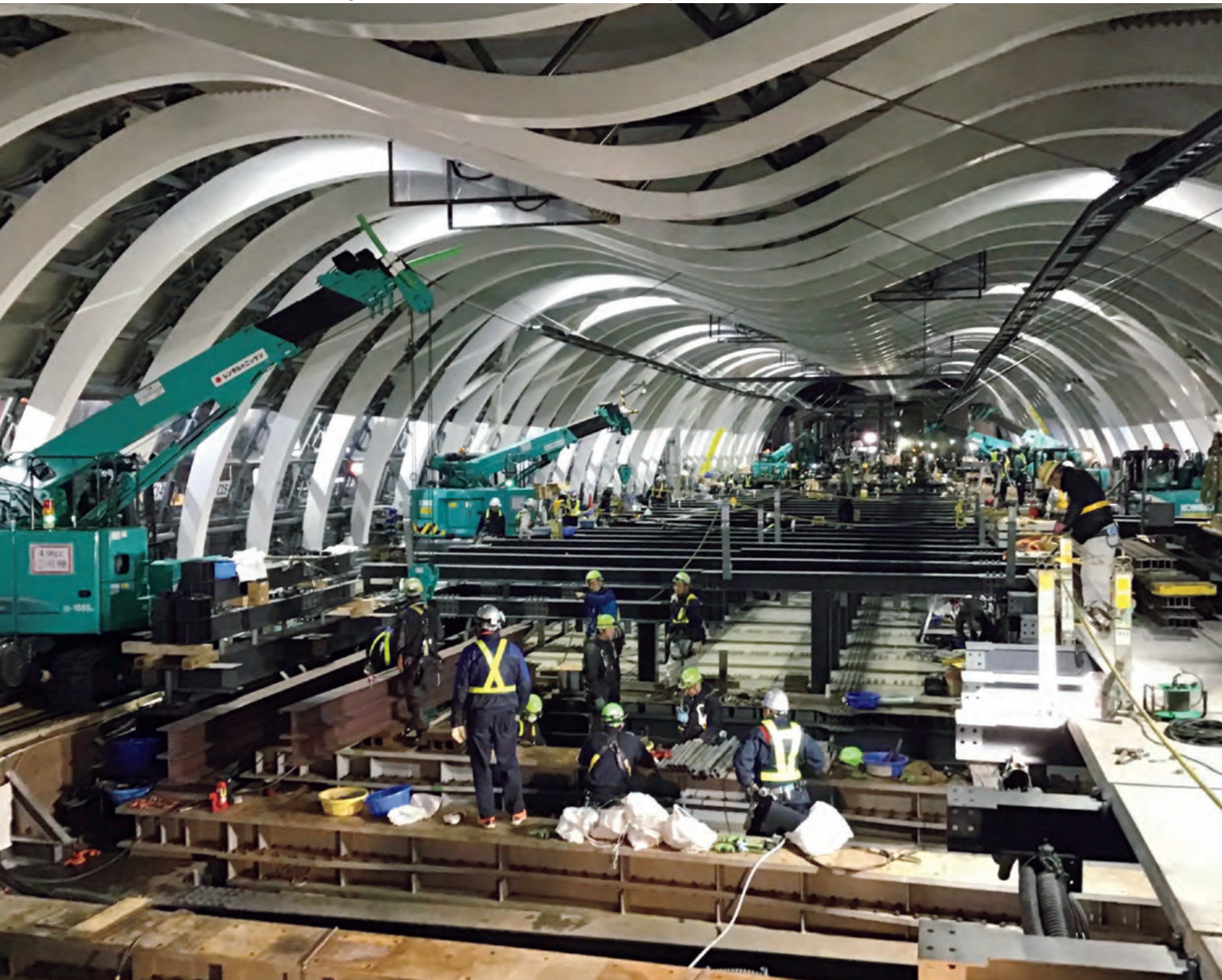
第3回線路切替のホーム桁架設状況 Platform girder installation for the third switchover of railway tracks
